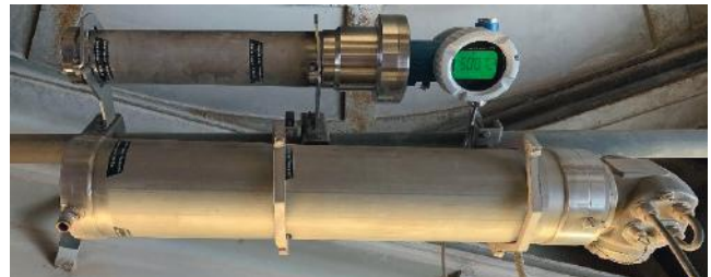
Figure 5: Field test results Parallel installation of the Gammapilot FMG50 and a water-cooled detector
