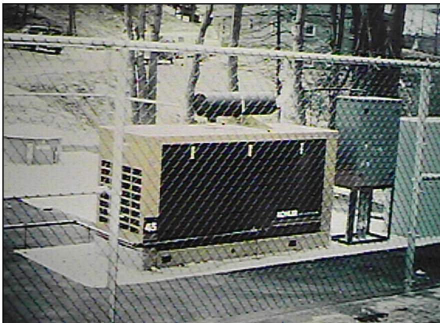
Permanently installed generator.
