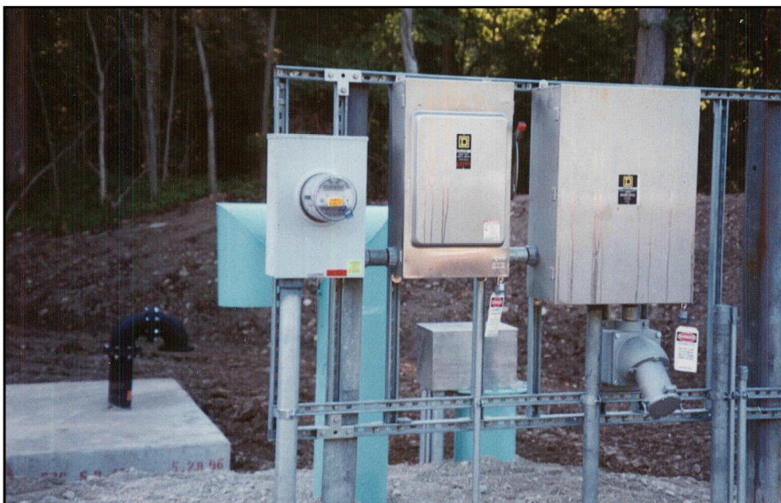
Typical “after market” switch gear and receptacle.
